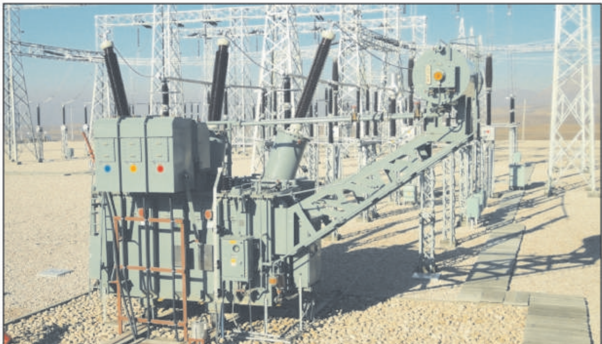
16MVA Power transformer at Aybak sub-station, Afghanistan
