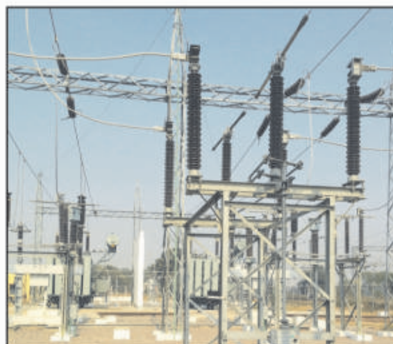
Sub-station in Lucknow-Mughalsarai Railway Electrification project
